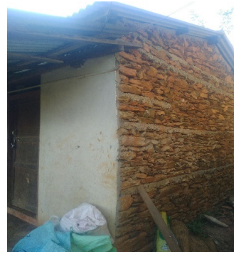
Figure 11: Poor roof to wall connection .
