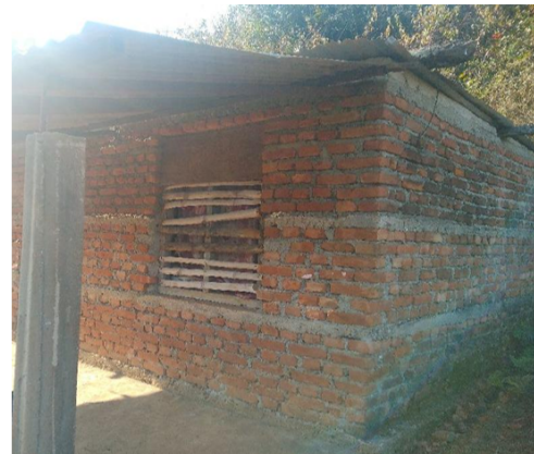
Figure 8: Inappropriate DPC results in mould formation.
