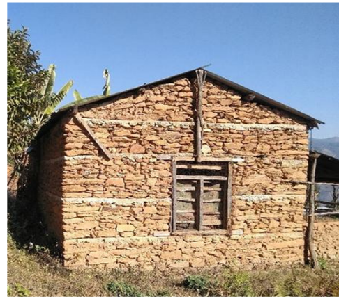
Figure 7: Improper band thickness and lack of gable band.
