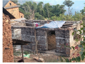
Figure 10: Reconstructed house without roof and visible vertical reinforcement.
