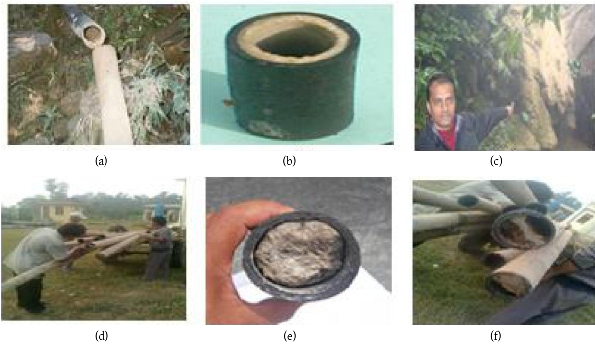
Figure 4: Scale formation problems due to high TDS and low pH. (a, b) Scale formation in outside and inside the pipe. (c) Scale formation in riverbed. (d, e) and (f) Scale formation in STWSSP - Mahendranagar.
