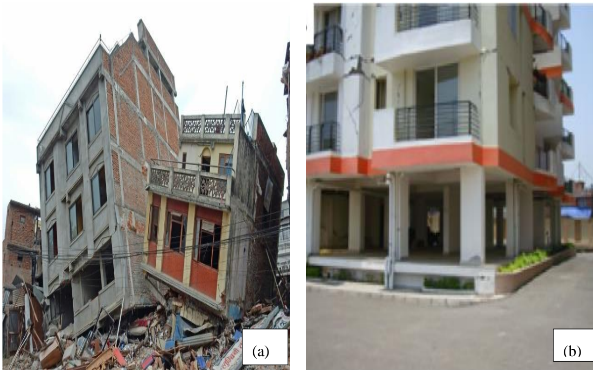
Figure 1. Soft Story Shear failure Gorkha earthquake (a) & (b) apartment in Nepal without infill in ground story [2]
