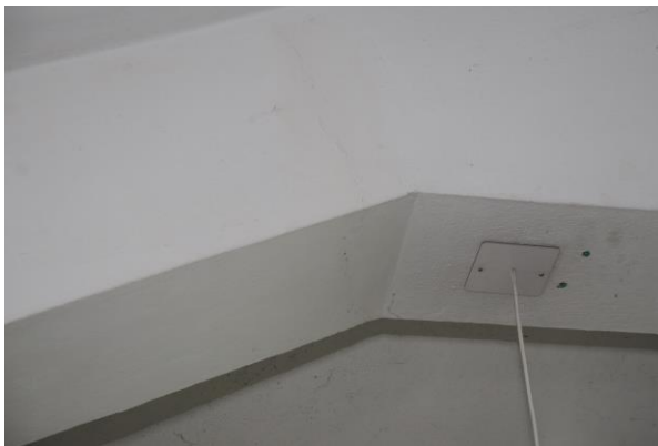
Figure 13: Cracks observed in inclined beam
