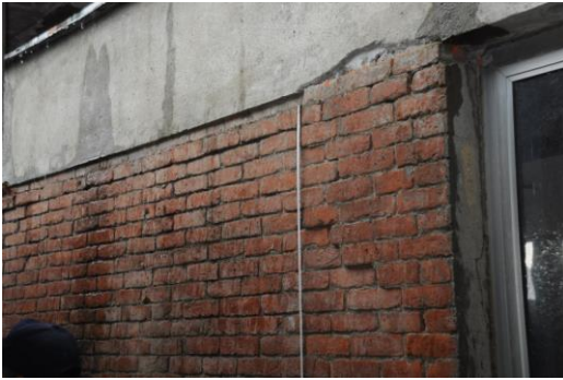
Figure 11: Out of Plane wall failure of cladding
