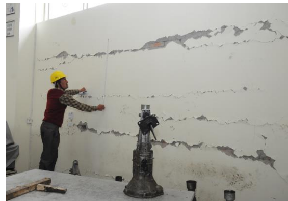
Figure 14: In plane wall cracks
