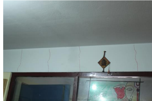
Figure 12: Minor Beam Cracks
