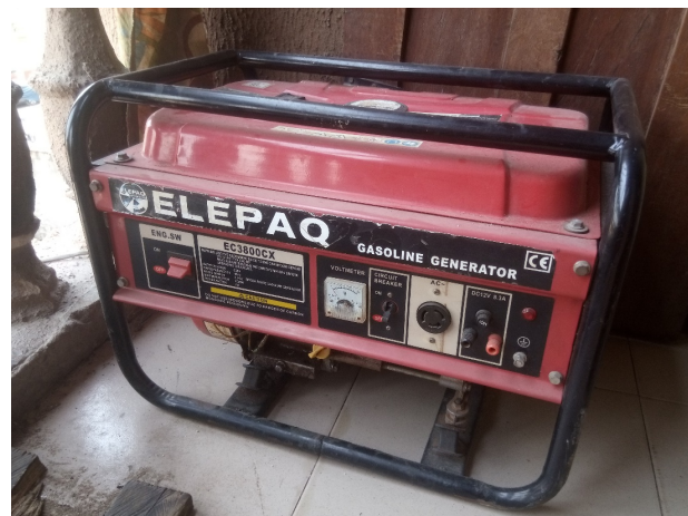
Figure 3: Elepaq gasoline generator.
